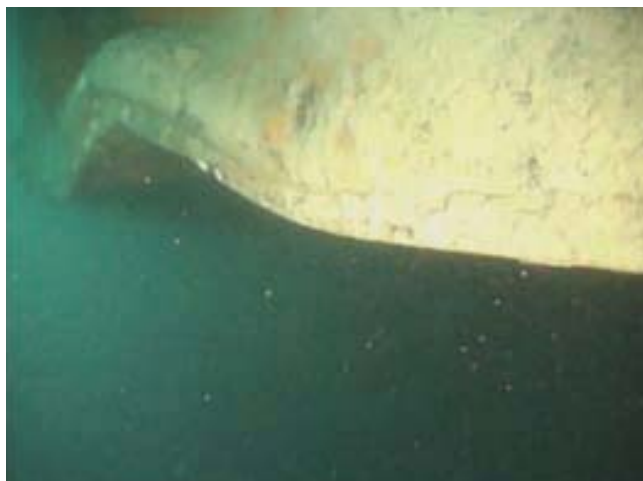
Figure 1 Deformation on bottom plate and side shell joint Slika 1 Deformacija na spoju donje i bočne ploče
