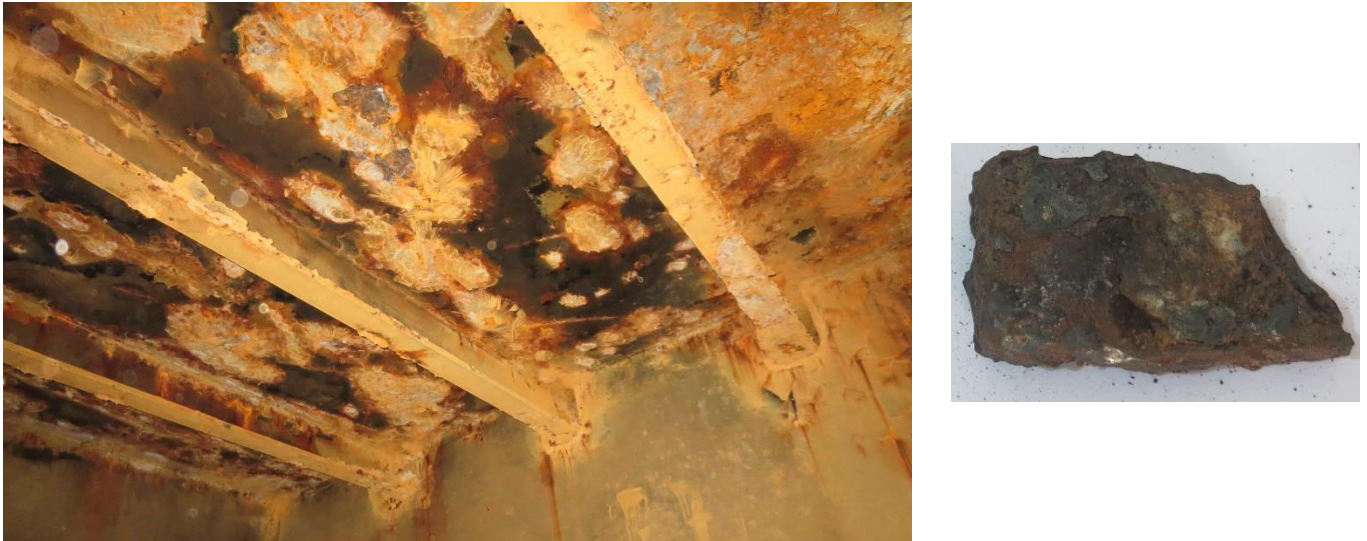
Fig. 2 Inner bottom plating: a) the bottom side of water ballast tanks, b) corroded piece of the inner bottom as a part of a fuel oil tank
