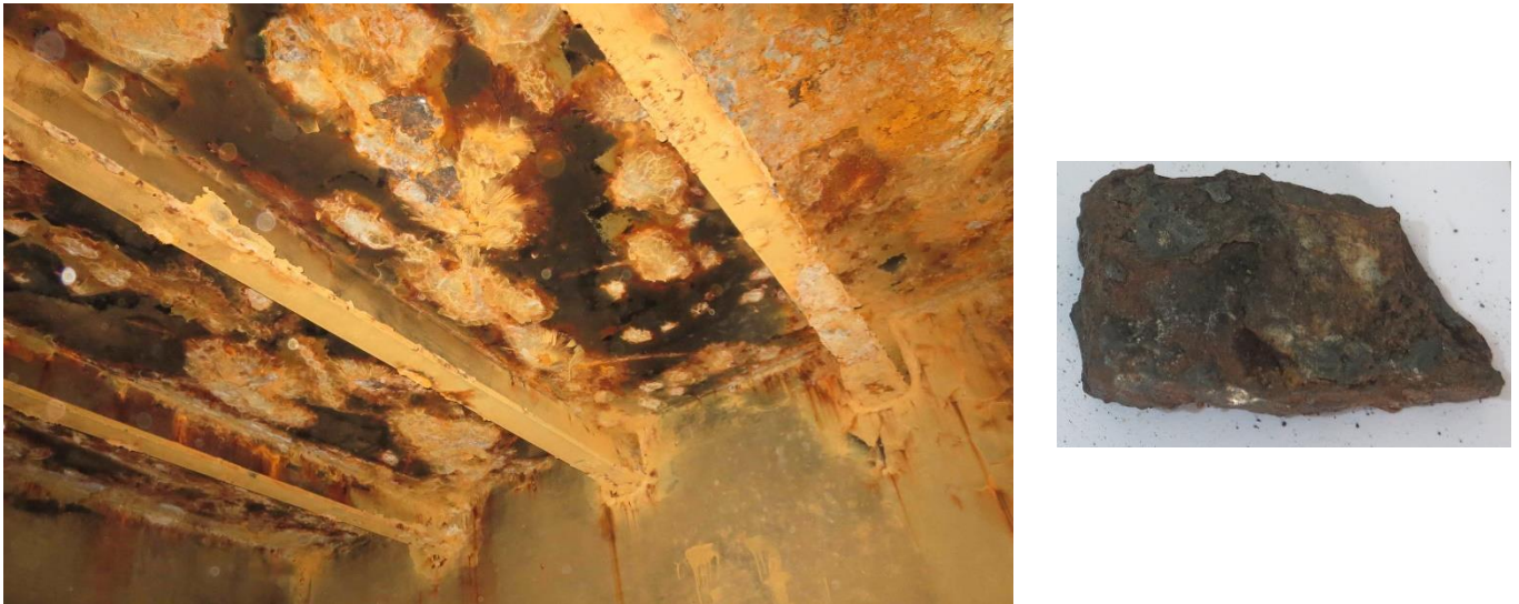
Fig. 2 Inner bottom plating: a) the bottom side of water ballast tanks, b) corroded piece of the inner bottom as a part of a fuel oil tank
